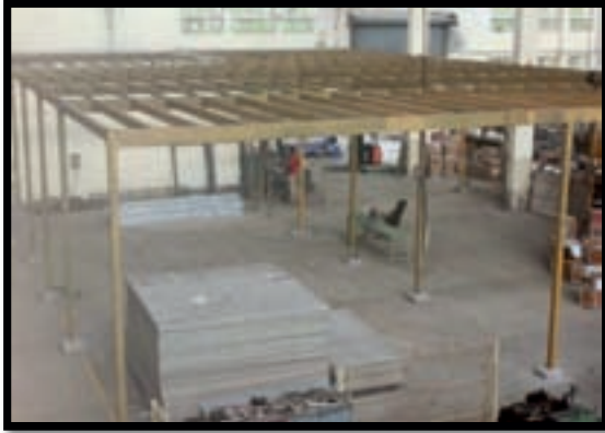
During the Structural Work being carried out at Integrated Facility for the Industrial Radiography Device (IFIR)
