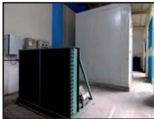
Chilled Air Plant of Low Temperature Irradiator
