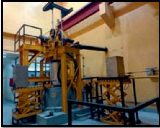
Hot commissioning of Low Temperature irradiator
