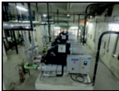
Fig. 9: Advance AC plant of LCL lab (screw chiller packages)
