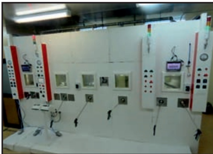
Fig. 2: Newly installed production facility for ^{131}\text{I} Capsules
