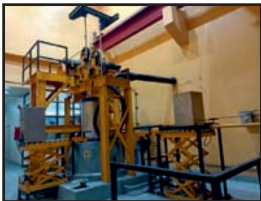
Low Temperature Irradiator Plant
